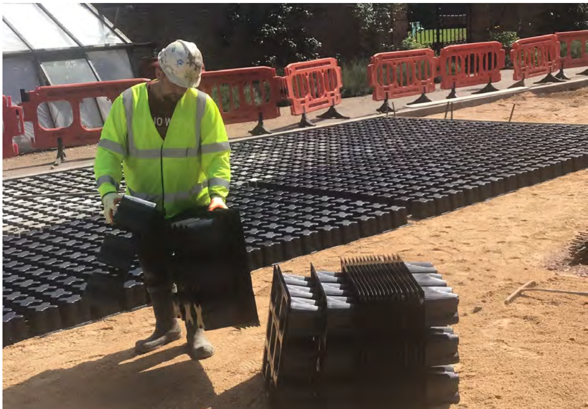
Fig. 12 Grasscrete GC2 void formers being removed from their nests, ready for installation
